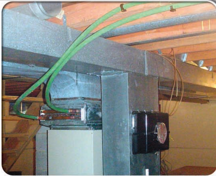
Forced Air Furnace
